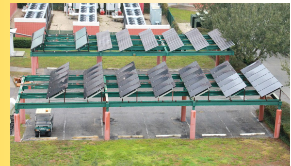
CERC's 20,000 watt solar photovoltaic electric charging station .
