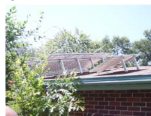
PV panels grace the roof of one of the tour houses.
